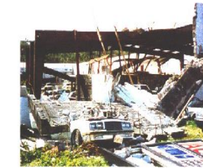
Poorly reinforced hollow-block walls can topple
