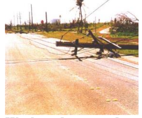
Weakened, ungued wooden power poles can break
